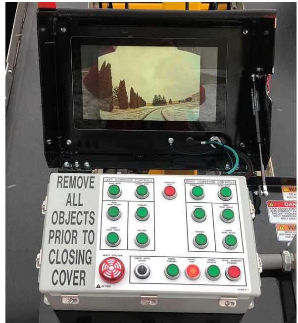
External Operator Control Box
